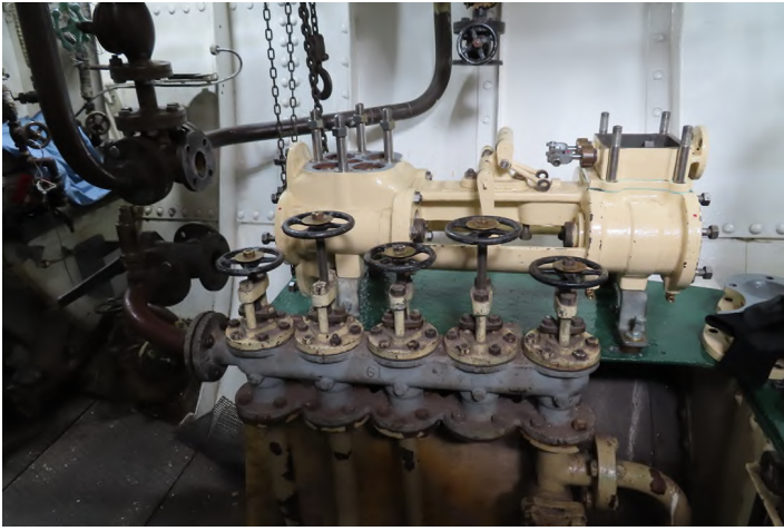
Partly installed, pipework yet to be attached, Oct 2021
