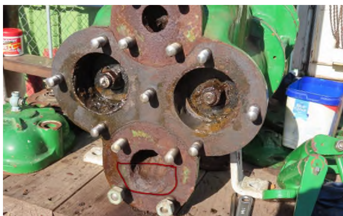
Red line marks significant corrosion on inlet port
