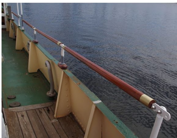
AMSA required safety rails, Nov 2020
