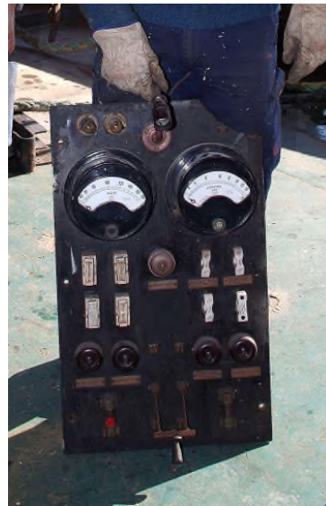
The original switchboard before reinstallation, for show only
